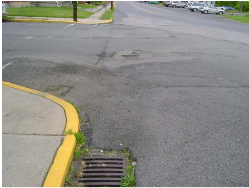
Figure C.16. Stormwater Inlet Located at Delaware Avenue and First Street
